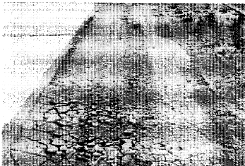
Figure D1 - Shoulder Deterioration
