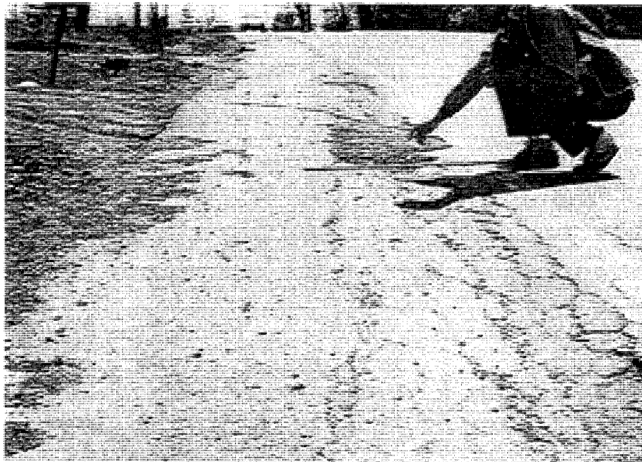
Figure D4 - Shoulder Deformation
