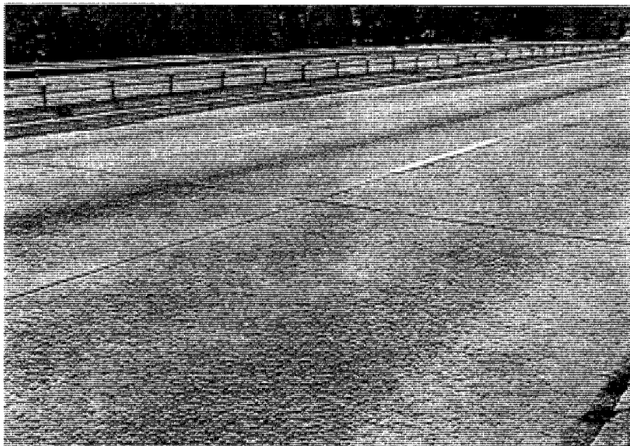
Figure B11 - Wheelpath Rutting
