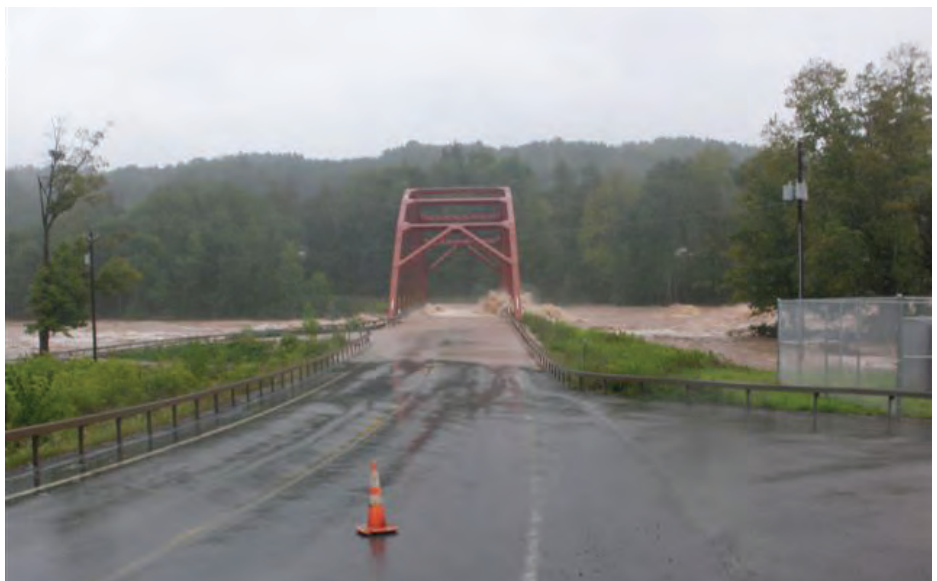
Severe flooding at this bridge below Gilboa Dam (2011) demonstrates nature's force on our infrastructure.
