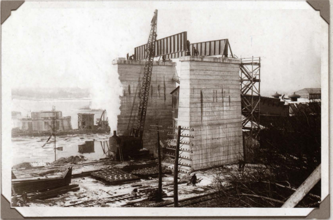
The bridge's first steel "stringers" are placed on top of concrete piers near the Black Rock Canal. The NYS Thruway now runs between these two piers.
