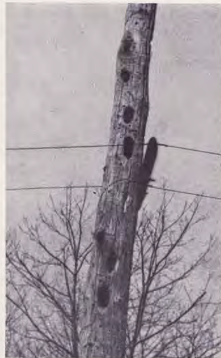
Excavations in electric utility pole shown here were made by pileated woodpecker and are typical of the damage now under study as reported in this article
